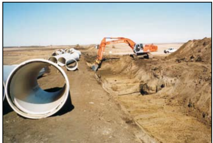
Exposed Gas Line: Secondary B North Branch
