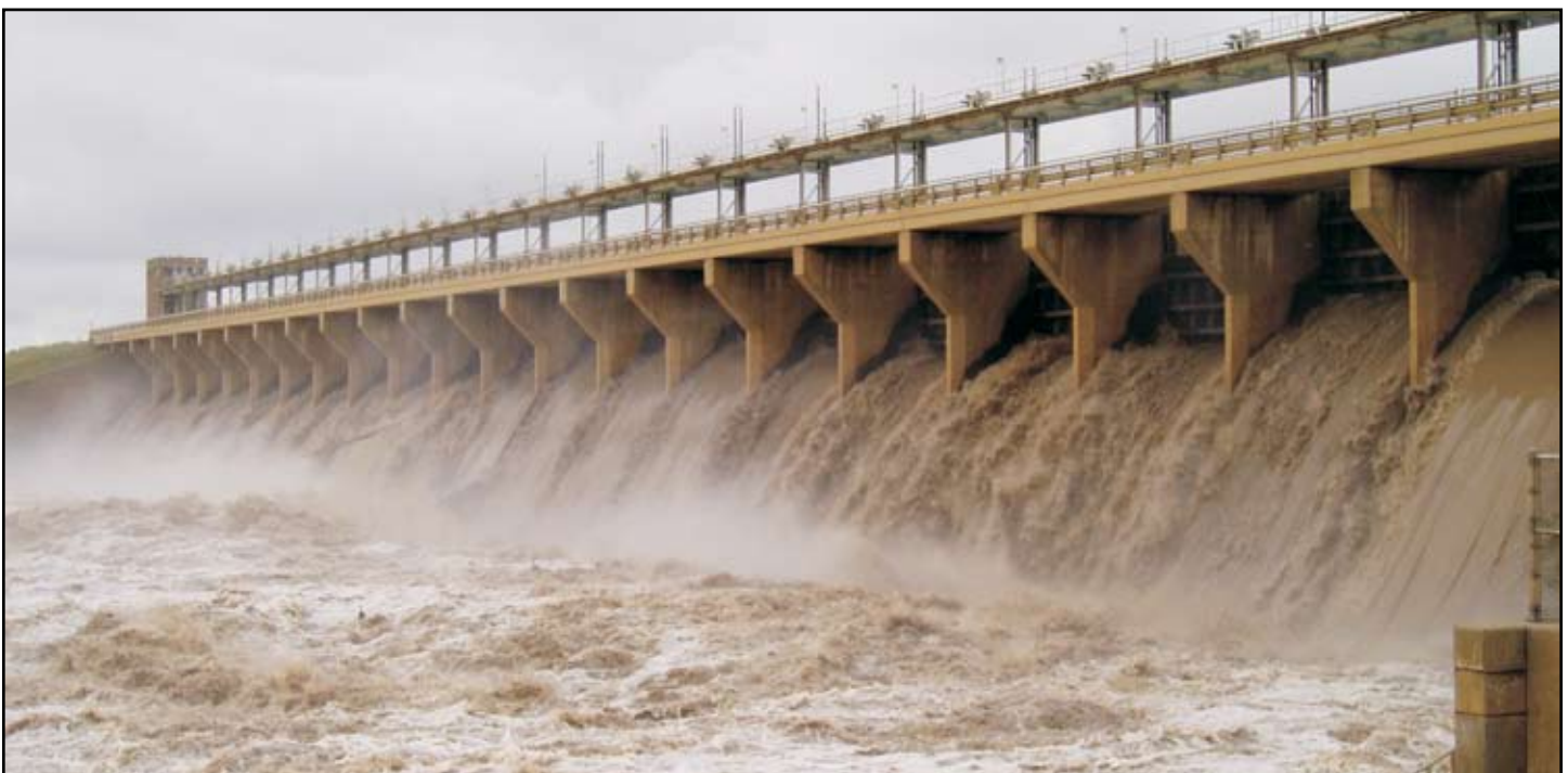
Bow River at Bassano Dam: 2005 Heavy Rainfall
