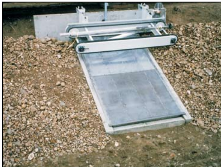
Trash Rack Cleaner: 26 Rolling Hills
